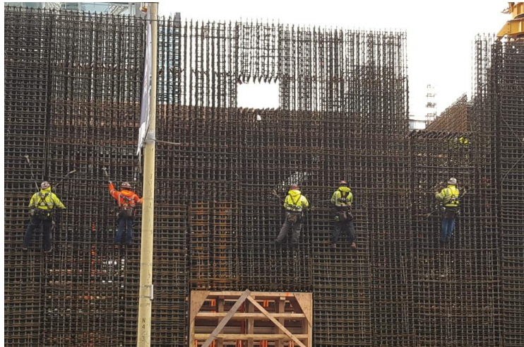
Figure 12 – Typical Steel Congestions
