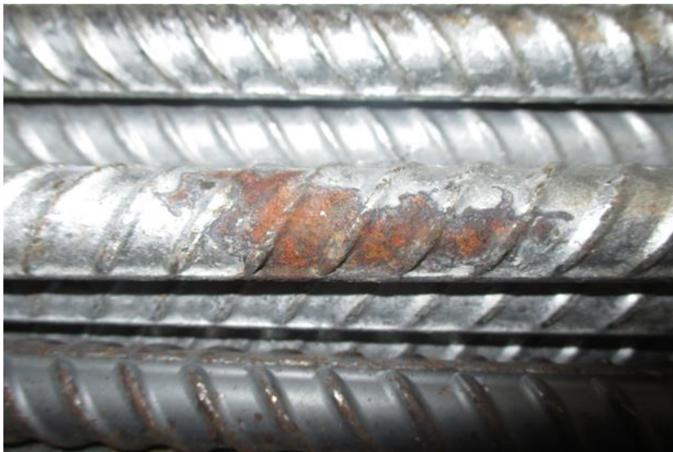
Figure 2.1: Lack of coating and exposed steel on A767 reinforcement. Bars with damaged coatings are not used in tests.
