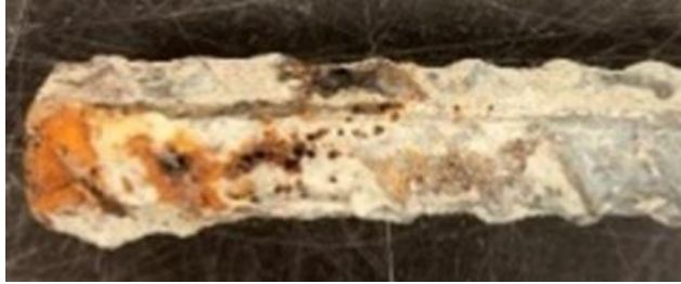
Figure 3.84: Conventional reinforcement from Cow Creek deck panel. Core taken at a crack location.
