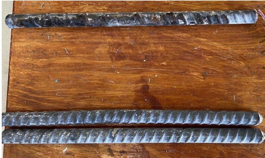
Figure 3.42: Cracked beam test. Specimen Conv-B-4 after 96 weeks of testing. Top mat (top) and bottom mat (bottom).
