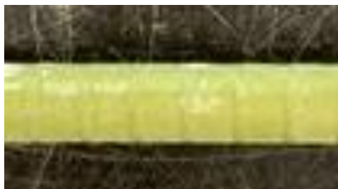
Figure 3.87: ECR from Cow Creek deck panel. Core taken in uncracked concrete.
